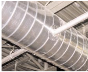
One of the many examples of pipe piercing duct; proving two objects can occupy the same space at the same time.
