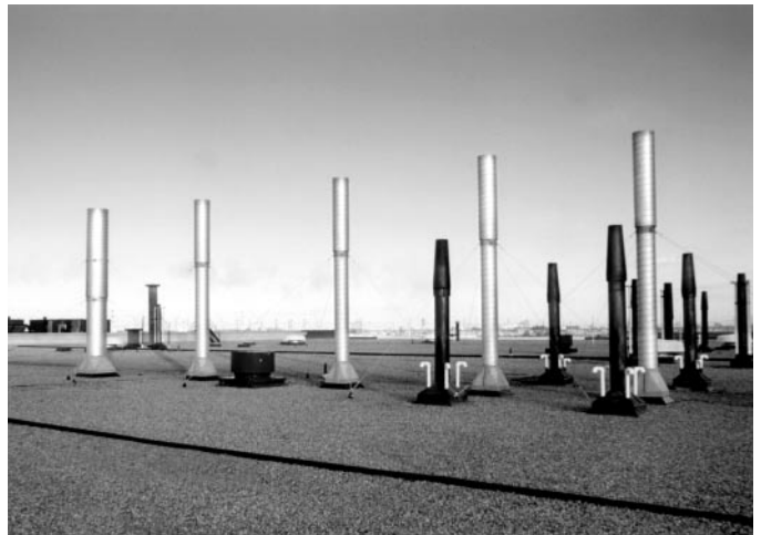
The innovative spiral duct, roof stack system, eliminated the need for extensive roof reinforcement.
