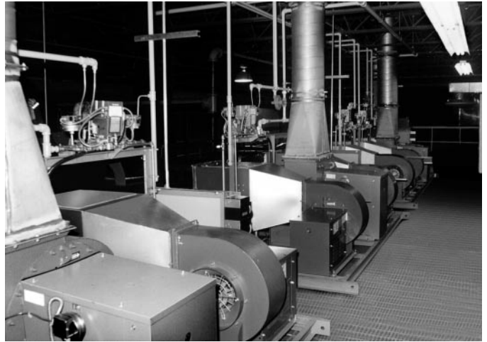
The new heating/drying system with its 100% efficient burners, installed above the newly assembled press line.
